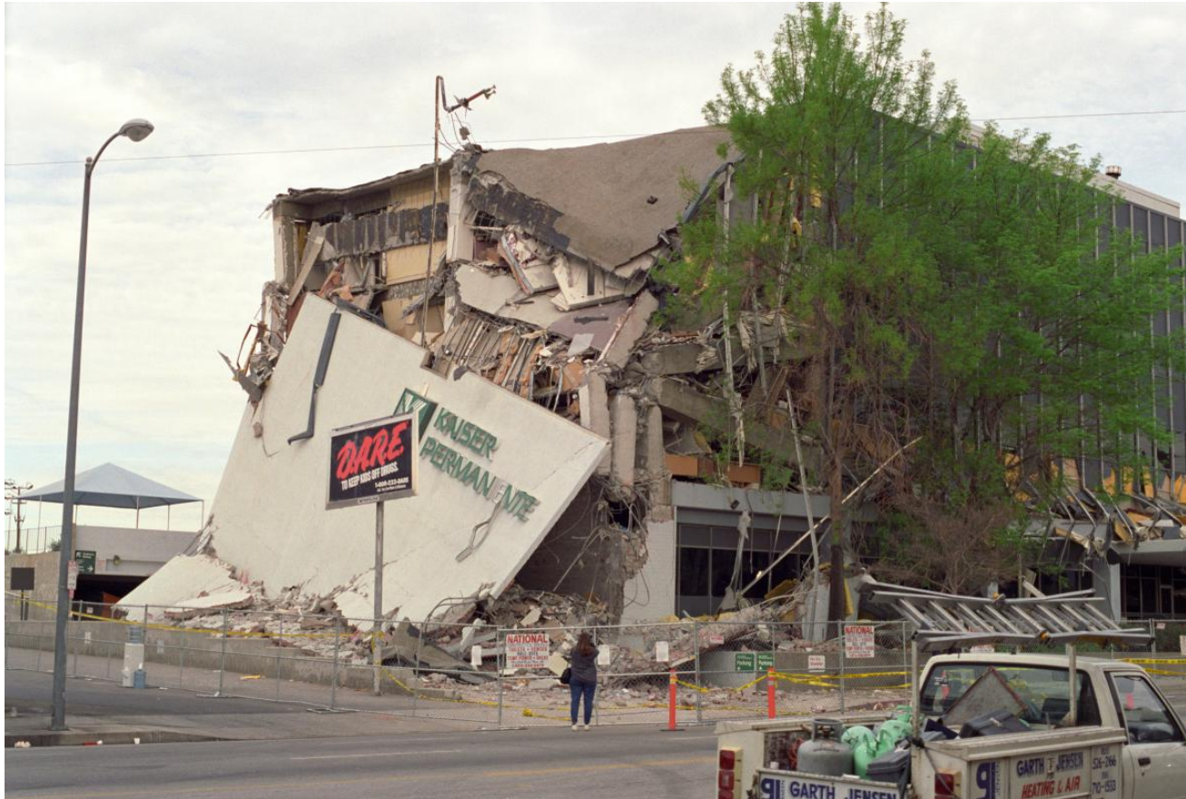
Photo: Gary B. Edstrom, Kaiser Permanente Building after the 1994 Northridge Earthquake. Public domain, via Wikimedia Commons.
