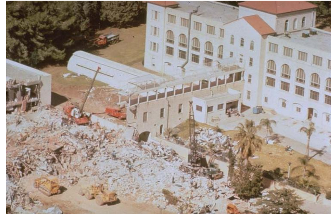
Photo: San Fernando VA Hospital, Sylmar – non-ductile RC hospital buildings that collapsed in the 1971 San Fernando earthquake, killing 49 patients and staff (USGS / LA Times).
